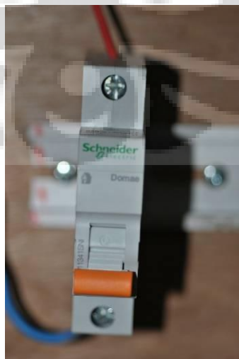
Gambar 3.22 Main contact breaker (MCB)
