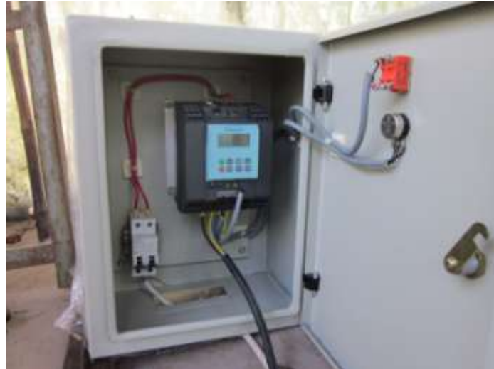
Gambar 3.12 Control Panel Blower Hisap IDF
