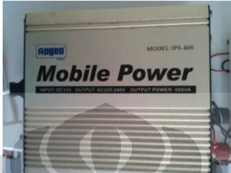
Gambar 3.30. Inverter merk Augen
