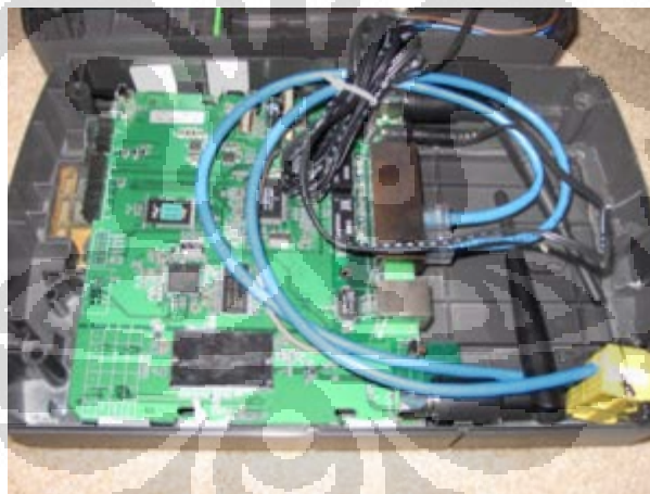
Gambar 2.13 Rogue Access Point Inside UPS [18]
