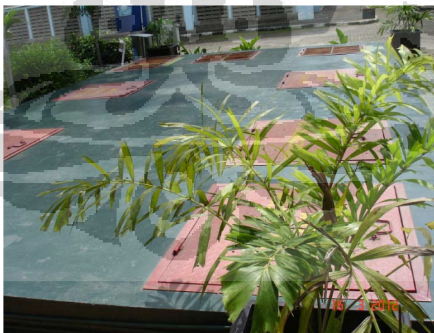
Gambar 3.4 Instalasi Pengolahan Air Limbah Pertamina Learning Center
