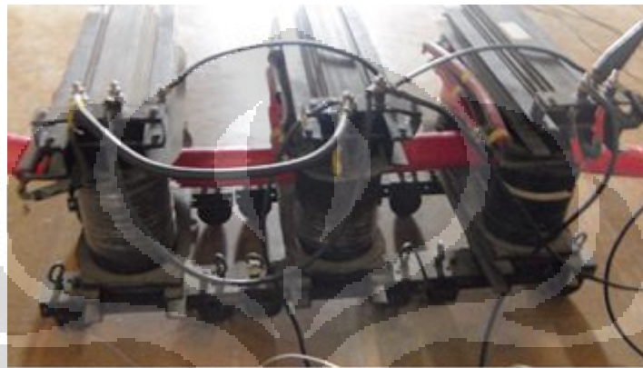
Gambar 3.2 Foto Current Transformer (CT)
