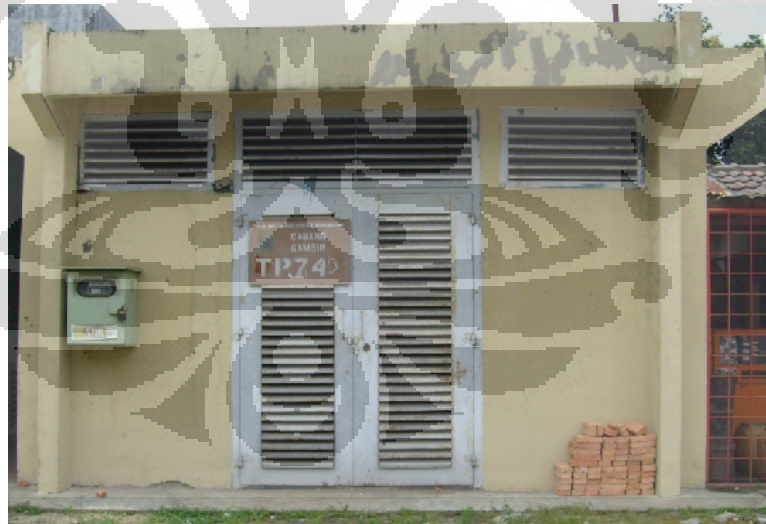
Gambar 2.8:Gardu Konvensional, Gardu Distribusi TP 74
