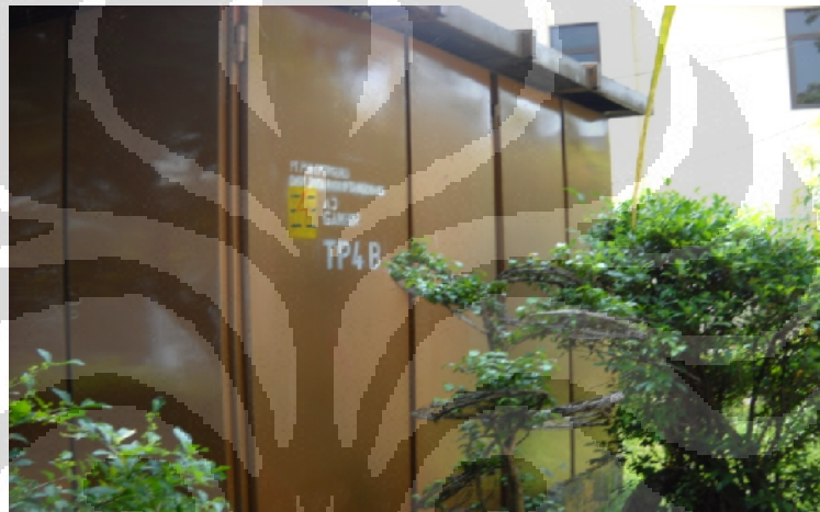
Gambar 2.9 : Gardu Besi, Gardu Distribusi TP 4 B
