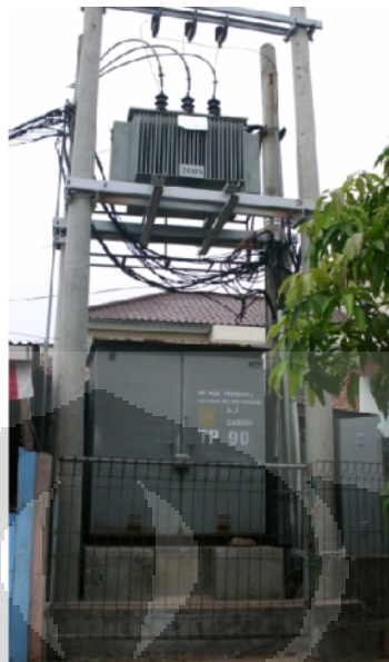
Gambar 2.10: Gardu Tiang Tipe Portal
