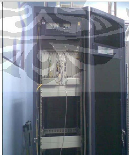
Gambar 2.9 Optical Line Terminal
