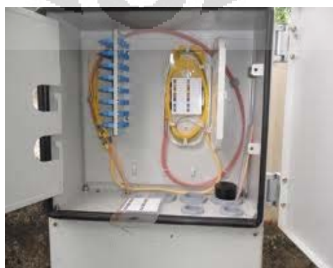
Gambar 2.12 Optical Distribution Point
