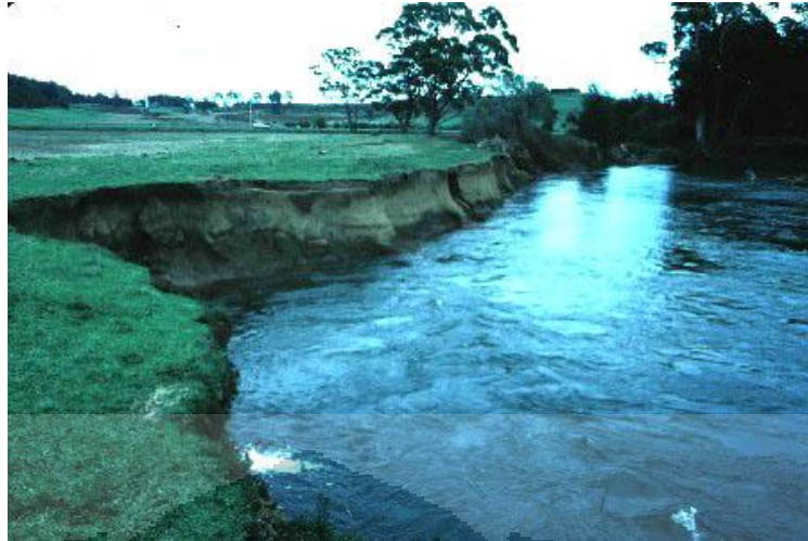
Gambar 2.7 Erosi Tebing Sungai
