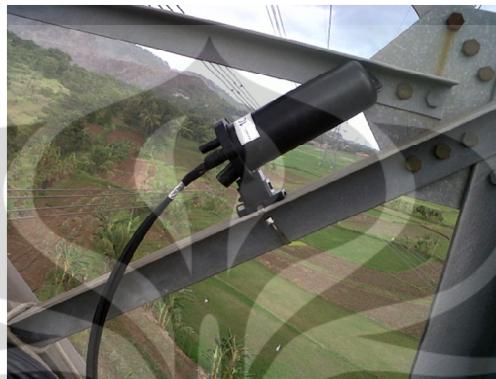
Gambar 3.4 Joint Box di Tower Sutet
