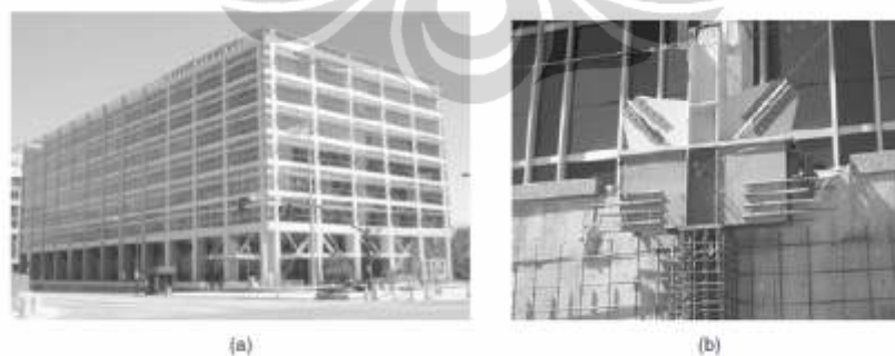
Gambar 2.18 Buckling restrained braces untuk rehabilitasi bangunan beton bertulang (a) Tampak Global (courtesy of SIE, Inc); (b) detail sambungan (courtesy Engineers & Associates, Inc)
