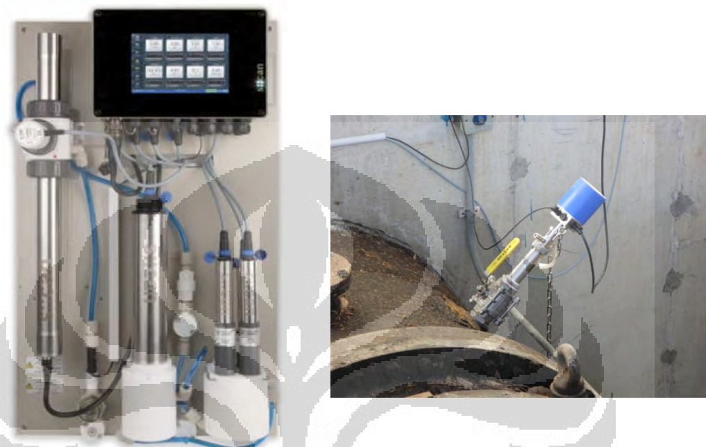
Figure 3.1 Example of sensor implantation in flow cell type (left) or in-pipe probe type (right)
