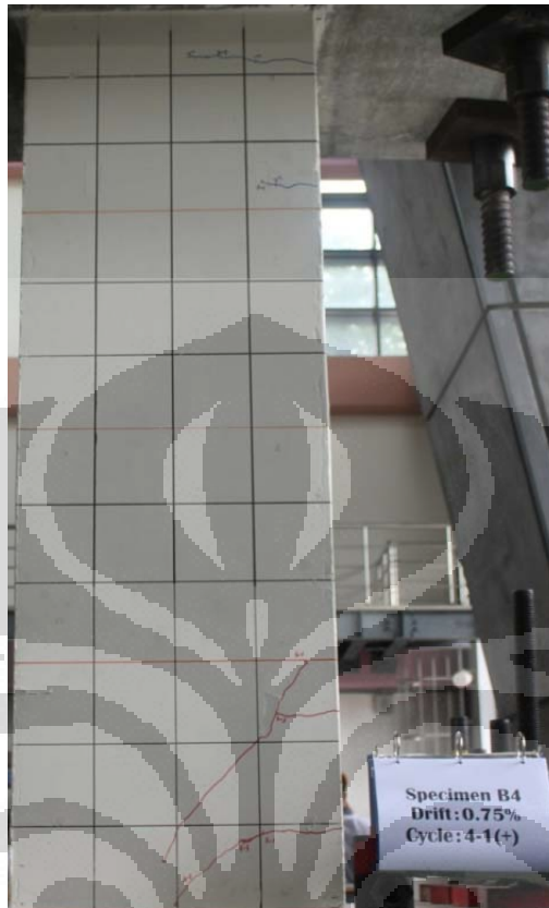
Figure 5.24. First shear crack at drift ratio 0.75 % width crack of 0.10 mm (west side).
