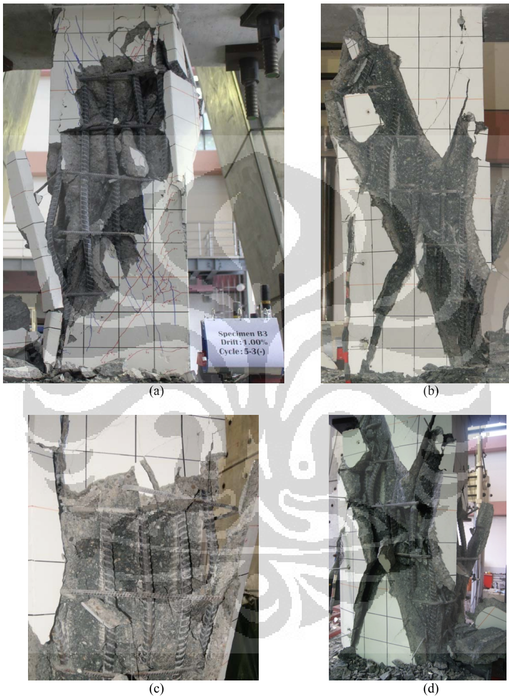
Figure 5.22 Final stage of column B3 (1.00 % drift ratio).
