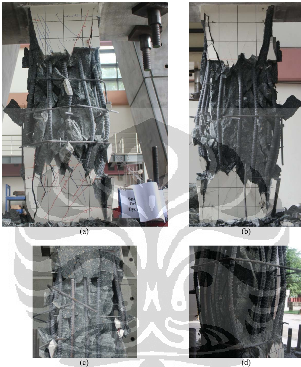
Figure 5.30 Final stage of column B4 (1.00 % drift ratio). (a) West side; (b) East side; (c) Failure of transverse reinforcement south side; (d) Buckling of lateral reinforcement at the upper of the column north-west side.
