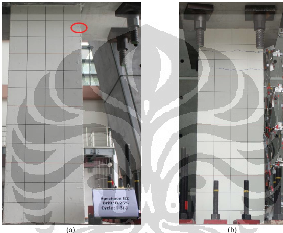
Figure 5.8 Flexural cracks during the initial displacements of column B2. (a) First flexural crack in west side; (b) First flexural crack in south side.
