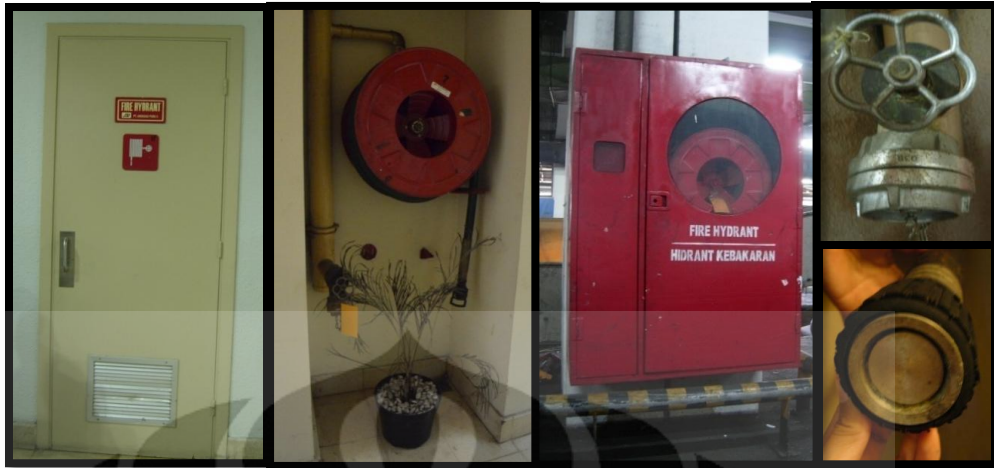
Gambar 6.13: Lemari hidran, hidran roll, hidran di Baggage Makeup , Siamese Connection , Nozzle
