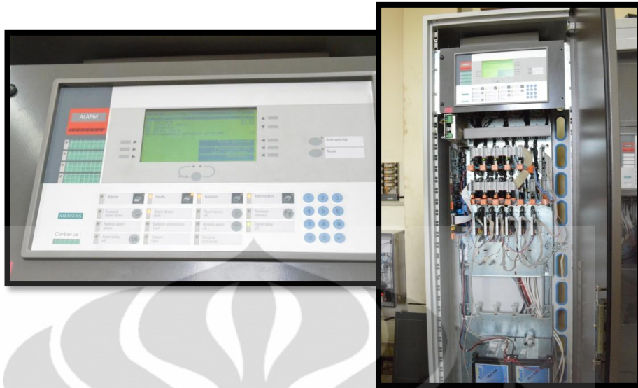
Gambar 6.5: Control Panel Alarm terminal 2
