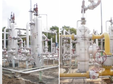
Scrubber SP Pasir Jadi
