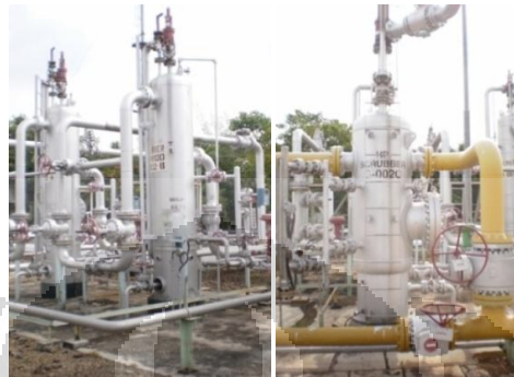
Gambar 6.7 Scrubber SP Pasir Jadi
