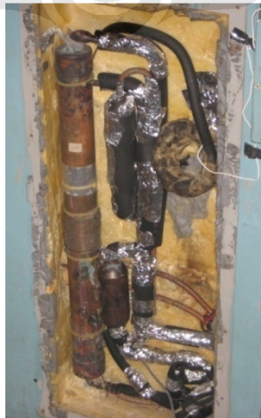
Gambar 3.3 Cascade heat exchanger
