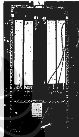
Flowmeter udara (Orifice)
