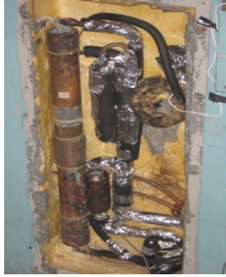
Gambar 3.4 Cascade heat exchanger
